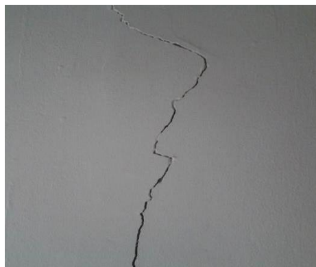
Fig 10: Crack of wall
