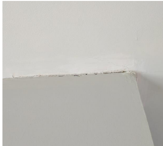
Fig 14: Air Gap between plastering & ceiling
